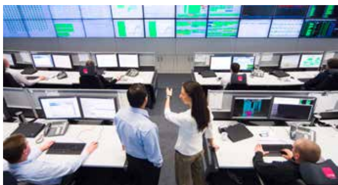
Fiducia control room at the Münster site
